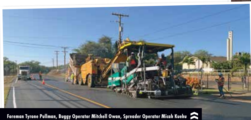
Foreman Tyrone Pullman, Buggy Operator Mitchell Owan, Spreader Operator Micah Kuehu and Screed Operator Joseph Kahaleanu complete milling and paving work on Hwy 460.
