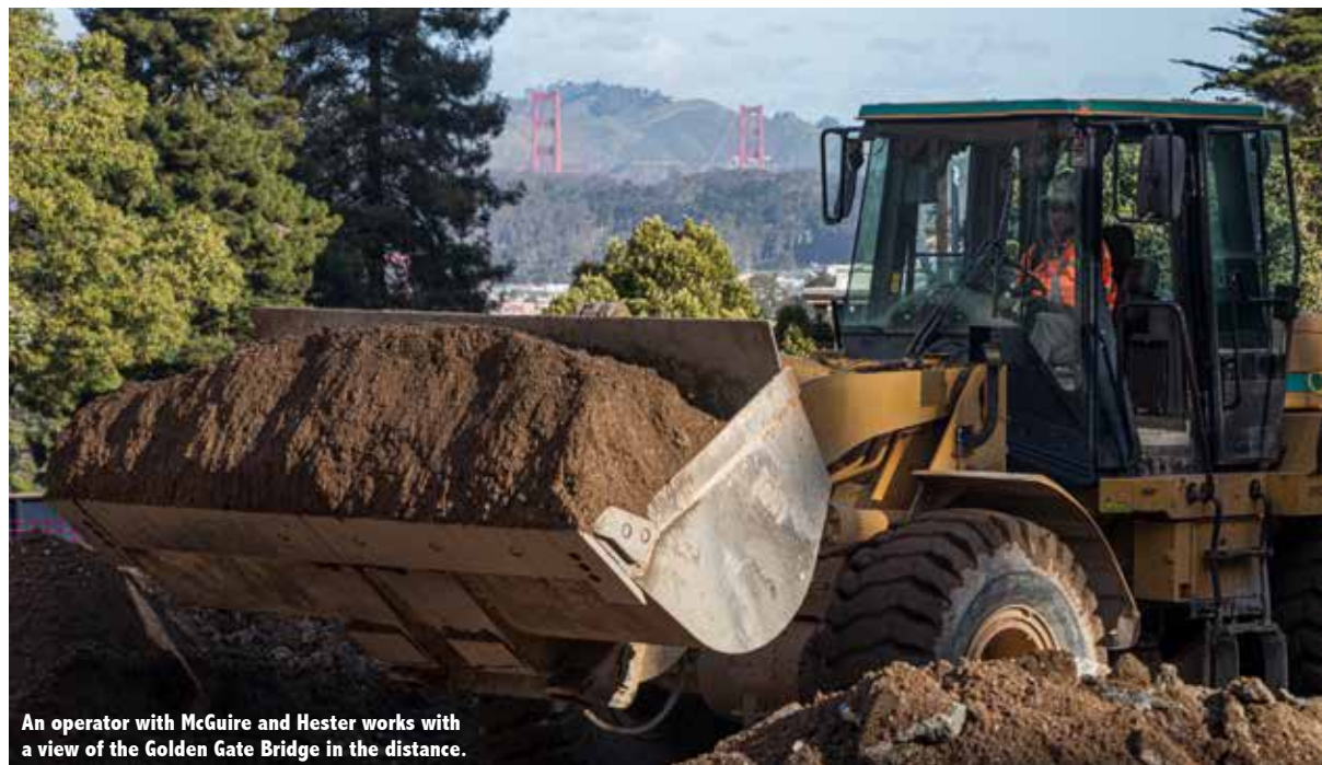
Ferma Corporation operators move dirt for a new research and academic building.
