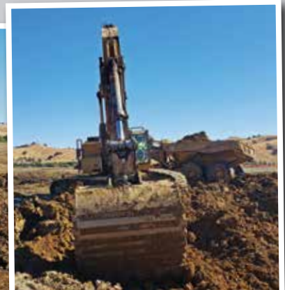
Dozer Operator Christina Solis and Excavator Operator Jose Alfredo work for Independent Construction.
