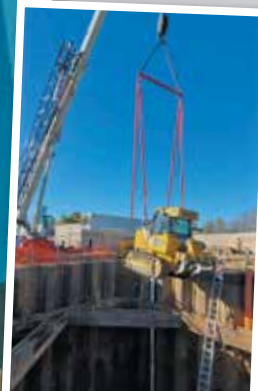
Operator Charles D. Newquist works on the Binney Junction project for Maxim Crane.
