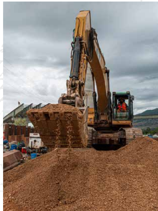
Excavator Operator Jesse Martinez backfills a bridge column on the West Davis Corridor project. (also right).
