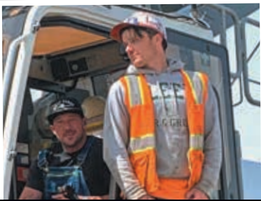
Peninsula Crane Operator Jason Vaux and Oiler Jared Holmgren work in San Bruno.
