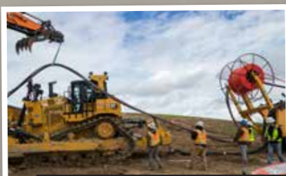
Local 3 members install a transmission line, as part of a renewable energy project in California's Central Valley.
