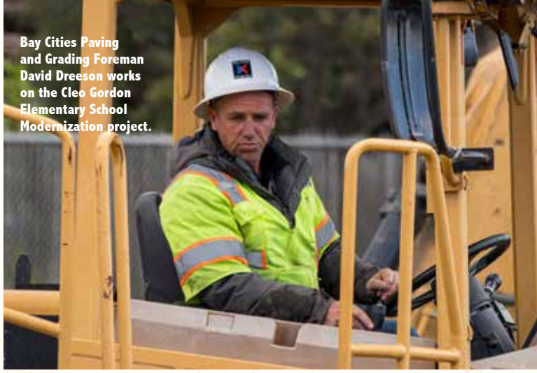
Operator Gus Carrillo works for Myers and Sons on the I-80/Hwy. 29 Separation Bridge project.
