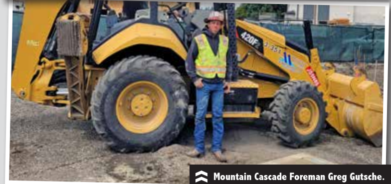
From left: Foreman Mike Dodgin, Operator Mason Buck and Gradesetter Myron Gonzalez work for KDW Construction.
