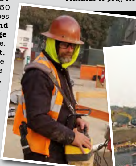
« Pump Operator Jon Fazier pumps concrete for Conco Pumping at the O Street project in Sacramento.
