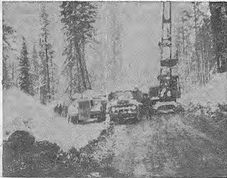
SNOW JOB —It is a bit rough going in the higher altitudes these days for Local 3 members. This view shows the brothers at work on the C. S. Phillips job on Highway 89 out of Meyers, Calif. On the job are: Buck Pelton, Bud Penno, Bob Corder, Dick Phillips, operators, Cal Hubbard and L. Christianson, oilers, and R. Phillips on drag line.
