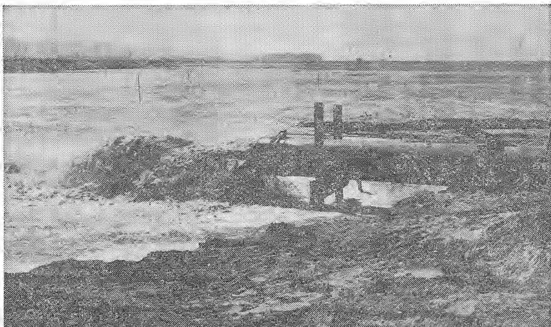
AND IT COMES OUT HERE: Water and sand are shown spurting out of a pipe laid from the storage basin to the fill area, pumped by a second dredge, Foster City DR 2, which floats in the basin. Parts of the Foster City tract are already being built upon. Some 18 million cubic yards of sand will be spread on the 2,600 acre tract to raise the level an average 4½ feet.
