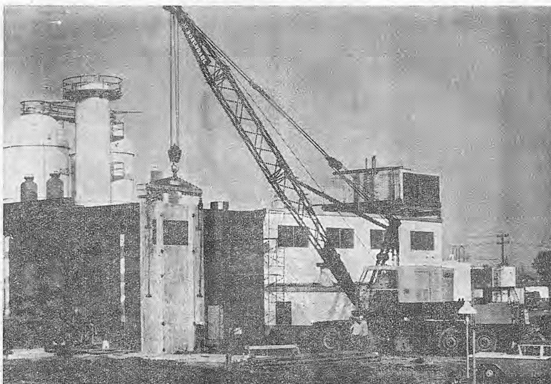
Rosendahl's new 65-ton Lorain truck crane on a job at the Airco Plant in Richmond. Bro. Stan Garber is the operator, with Bro. Bob Pacini as his oiler.
