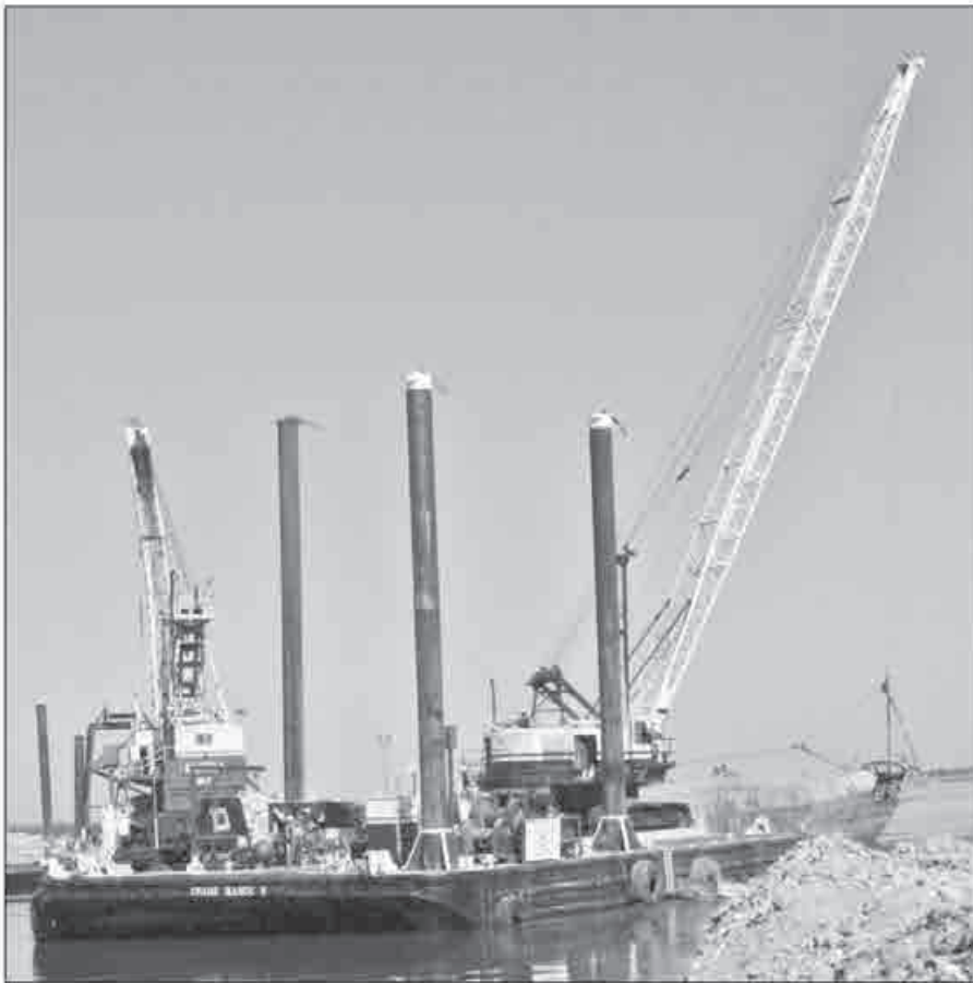
Crane Barge 8 and Derrick Barge 24 are put to work to repair the levee break.
