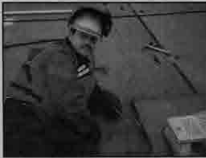
First-period Heavy Duty Repair Apprentice Christopher Fernandez gets ready to make a few passes on the deck of a barge while employed by Kiewit Pacific at the Vallejo laydown yard.
