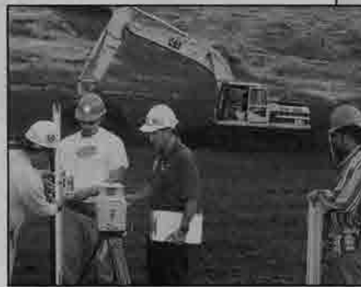
From left: Checking out the laser are apprentices Angel Julian, Robert Rust-Sipili, Instructor Alan Kumalae and apprentice Severino Nahinu Respicio. Apprentice Adran Hoopai operates the excavator.
