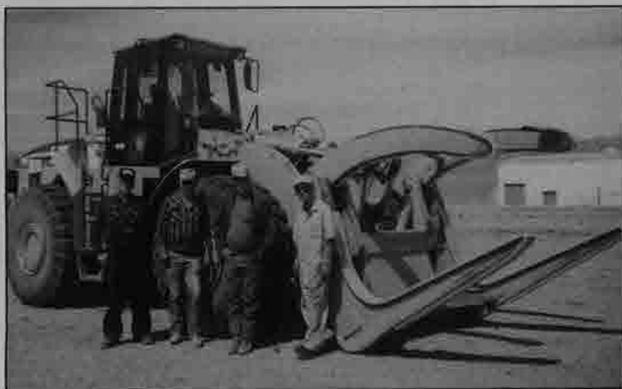
Operators John Zaruba, Roger Harwood, John Rogers and Earl Garden at the pipeline project in Tooele.
