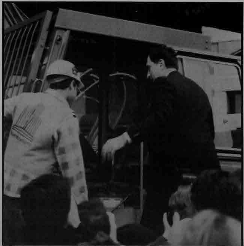
San Francisco Mayor Art Agnos climbs into an excavator equipped with a breaker attachment to take the ceremonial first whack at the quake-damaged Embarcadero Freeway.
