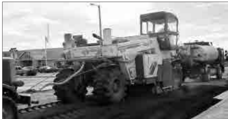
Western Stabilization recently reconstructed Franklin Street from Cypress to Oak Street using a method known as cold-foam injection.
