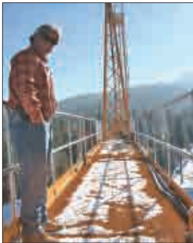
Member Bruce Maes checks out the snow level on his counter jib. Maes said the last snowstorm piled 1.5 feet of snow on his crane, which had to be shoveled because of the enormous amount of weight it added to the back of the crane.
