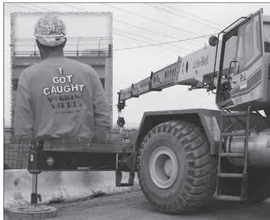
Local 3 member Charlie Ambler was "caught" on the job at Douglas Boulevard wearing this shirt, designed with safety in mind by R&L Brosamer . Ambler operates a 65-ton hydrocrane for the company.
