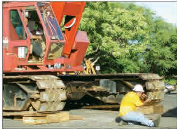
Business Rep. Danny Padeken and Crane Operator Walter V. Keamo work together on the WCHC jobsite.
