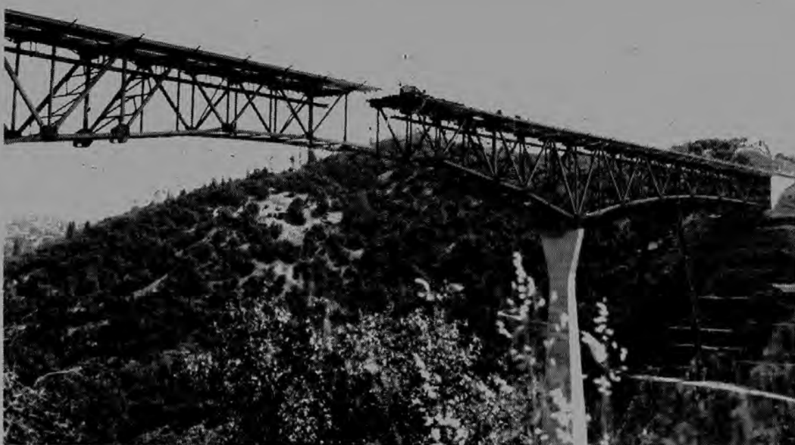
7,200 TONS OF STEEL (top photo above) forming the new Auburn-Foresthill Bridge was put together with the help of Local 3 brothers Floyd "Slim" Ciachon, Kenny Bettis, Eules Grigsley, Gary
