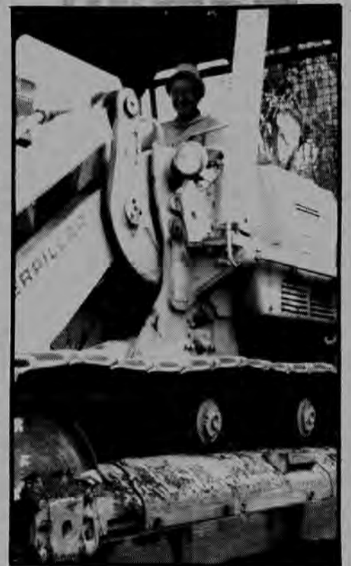
Track loader operator Isaac Inouye works for Les Hirahara on the Hana airport job.
