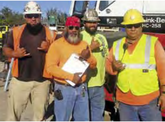
From left: Hydraulic Monitor Operator Harry Au, Crane Operator Daniel K. Kahumoku, Welder Ikaika Eulitt and Oiler John W. Kahoonei III work for Frank Colluccio on the sewer tunnel from San Island Wastewater Treatment Plant to Pier 1.
