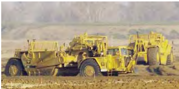
At the River Islands project, members with Independent Construction perform some de-watering to keep the job moving.
