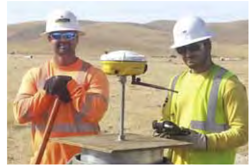
Josh Robinson and Jon Castaneda work for M.A. Mortenson on the Quinto Solar project.
