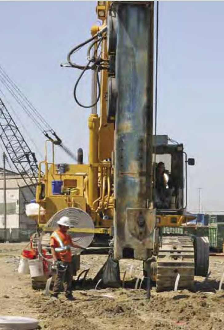
Operator Tim Goss and first-step Apprentice Max Phelps work for HB Wick Drains.
