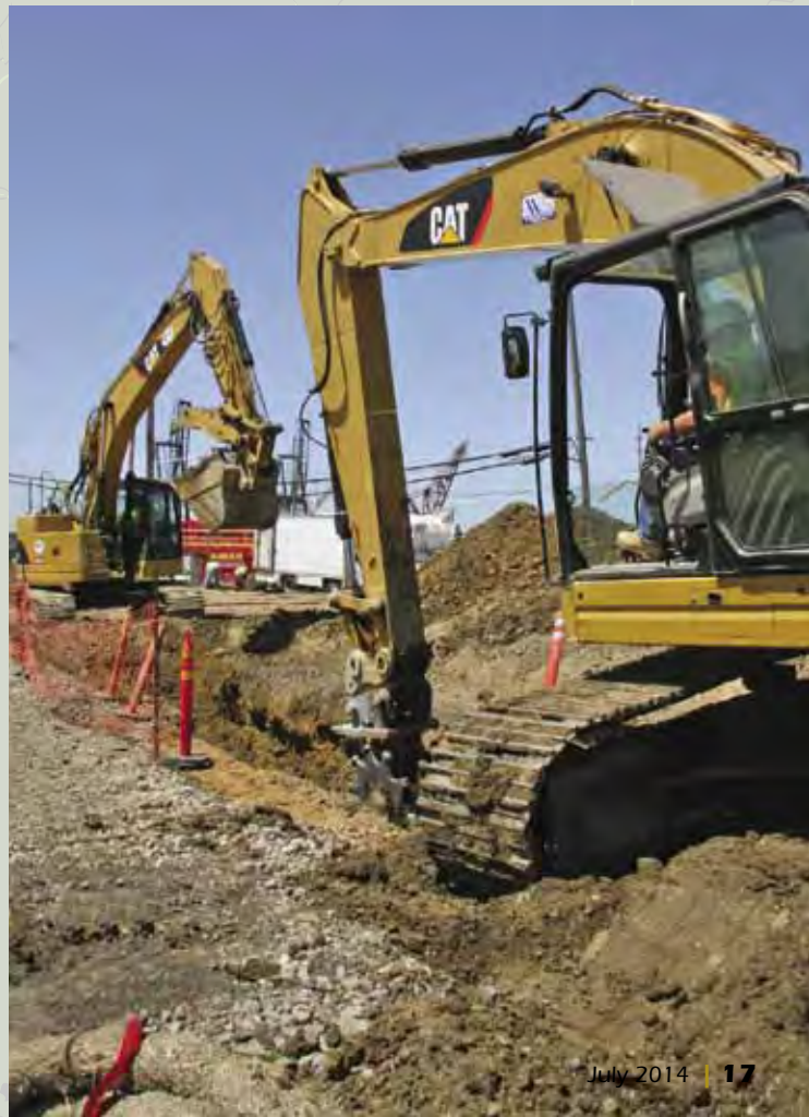
From left: Top Grade excavator operators Alfredo Alfaro and Brad Chitwood perform the utility abandonment.
