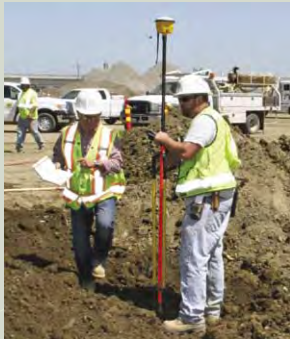
Inspector Robert Uribe talks to Gradesetter Scott Jennings about elevations and locations on the project.
