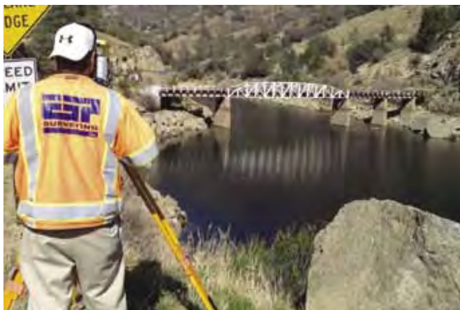
ESP Party Chief Sam Espinosa sets up along the San Joaquin River as part of the bridge-replacement project on Italian Bar Road.
